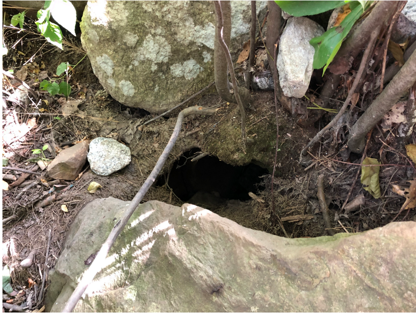
Photo 3: The inlet to the culvert can be seen behind a large rock. The culvert is \frac{1}{2} filled with years of sediment buildup from the surrounding BVW.
