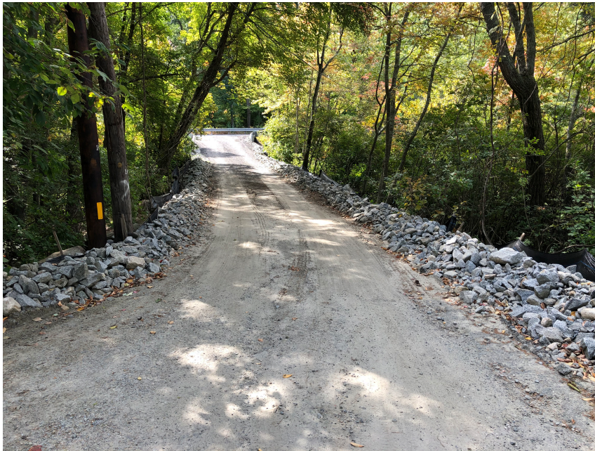
Photo 4: A view of the improved gravel driveway and Hartford Avenue West in the distance. Rip rap and silt fence can be seen at the edges of the driveway, preventing sediment from reaching the BVW.
